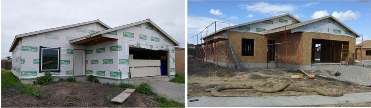
Figure E4. The two ZNE homes under construction in 2020. One was an all-electric home, while the second used a tankless combined space and water heating system. Both were monitored and used for validation of building energy models in this phase of the project.
