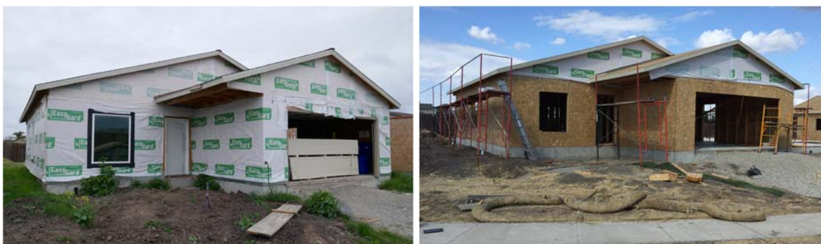
Figure 9. The two ZNE homes under construction in 2020. One was an all-electric home, while the second used a tankless combined space and water heating system.
