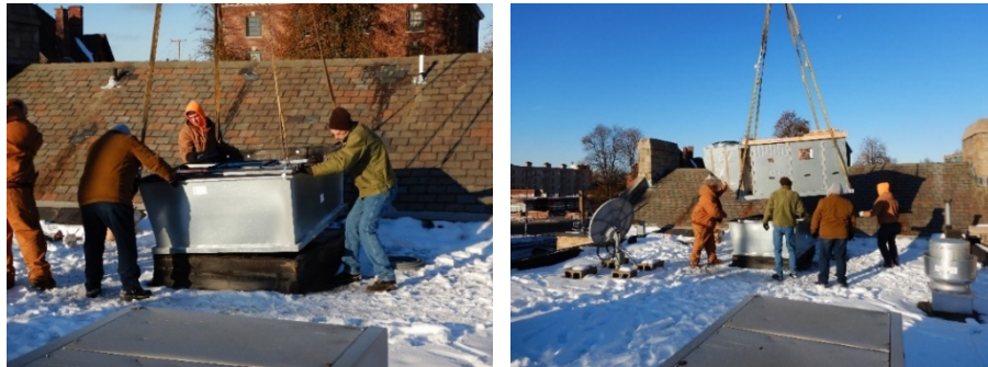
Figure 3. A custom transition curb was to install the PGHP with the existing rooftop curb and interior ductwork.
