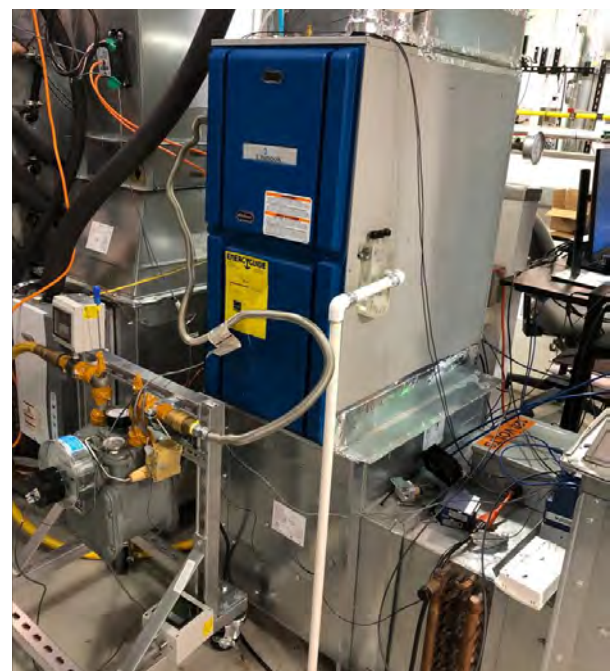
Furnace test bay with final modulating furnace installed for testing.
