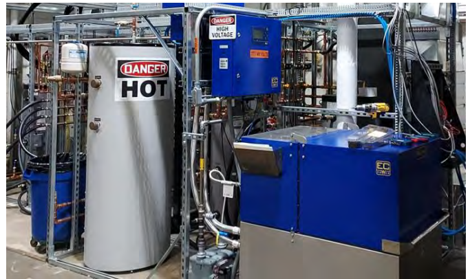
The mCHP integrated system indoor installation.
