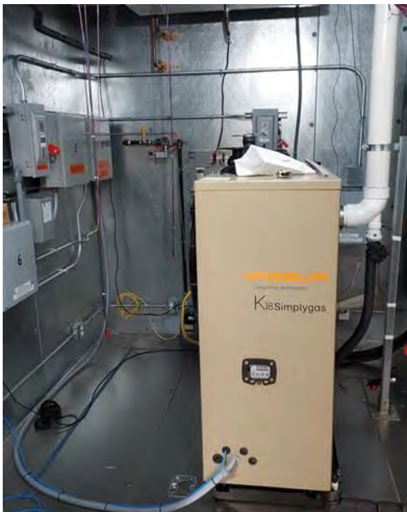
A prototype North American Robur K18 GAHP installed inside a laboratory environmental test chamber
