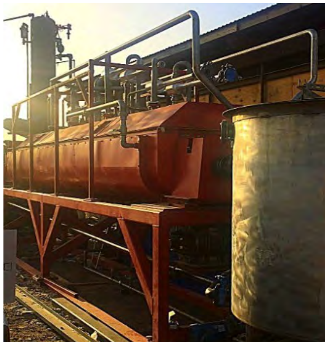
Thermo-Vacuum Dryer of 100 tons per day capacity in previous UTD project 2.17.B
