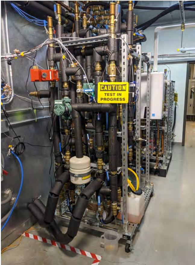
Completed laboratory test stand.
