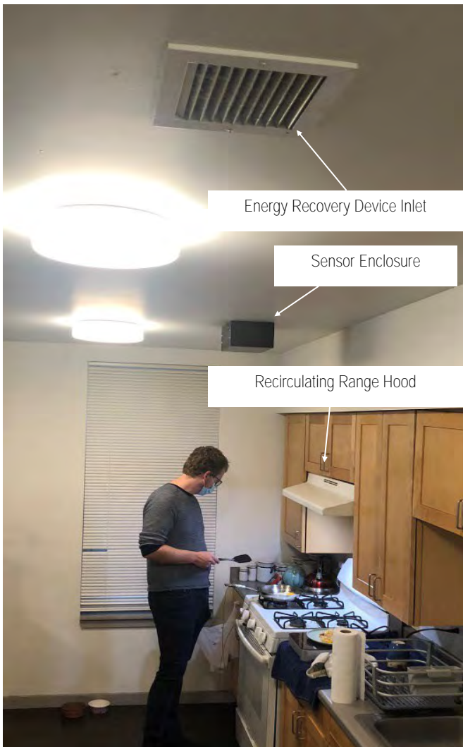
IAQ sensor installed in kitchen with an energy-recovery ventilator.
