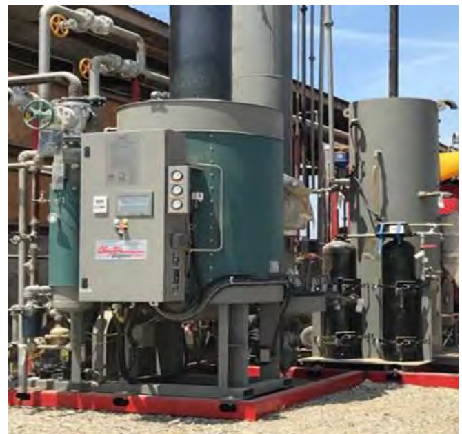
Thermo-Vacuum Dryer of 100 tons per day capacity in previous UTD project 2.17.B.
