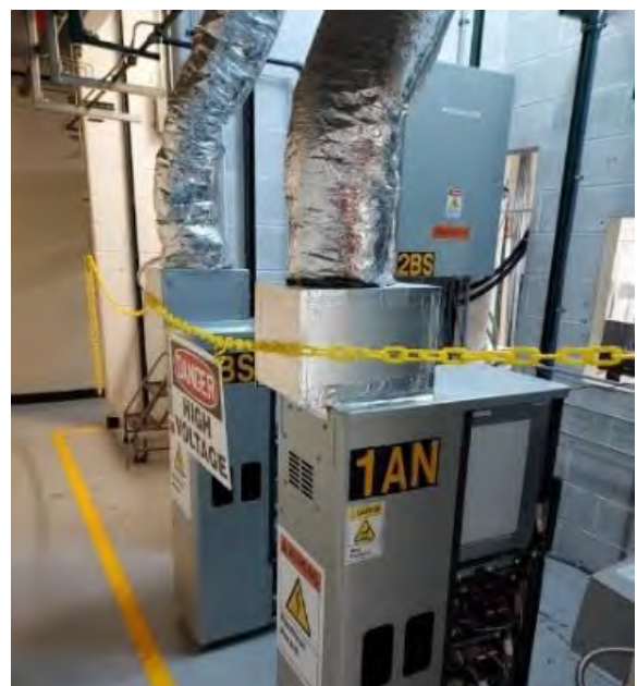
AISIN SOFCs installation at research laboratory
