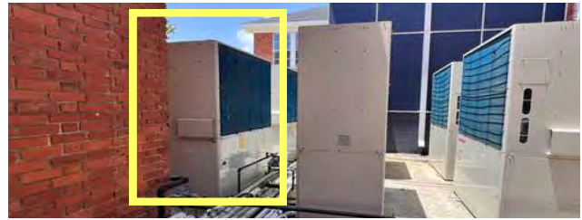
One of seven two-pipe GHPs installed at Pike Road School in Alabama.
