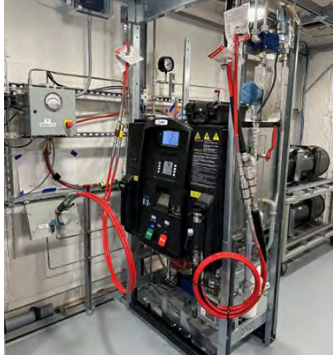
The fully installed ANGI dispenser
