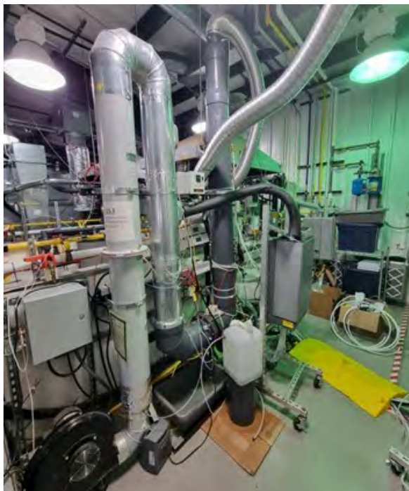
The regenerator tower
