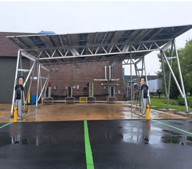
The mCHP integrated system outdoor installation.
