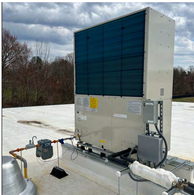
Example of a Yanmar Gas Engine Heat Pump being analyzed, with a gas meter to monitor gas consumption
