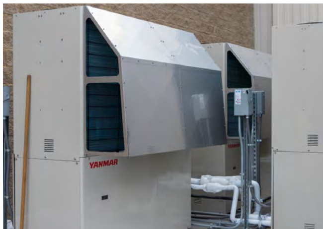
One of six GHPs installed at the Lawrenceville Public Works facility in Georgia.
