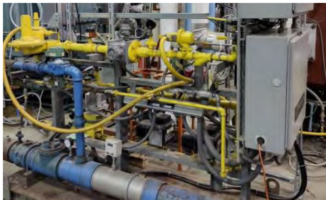
Air-fuel skid assembly for H2 operation
