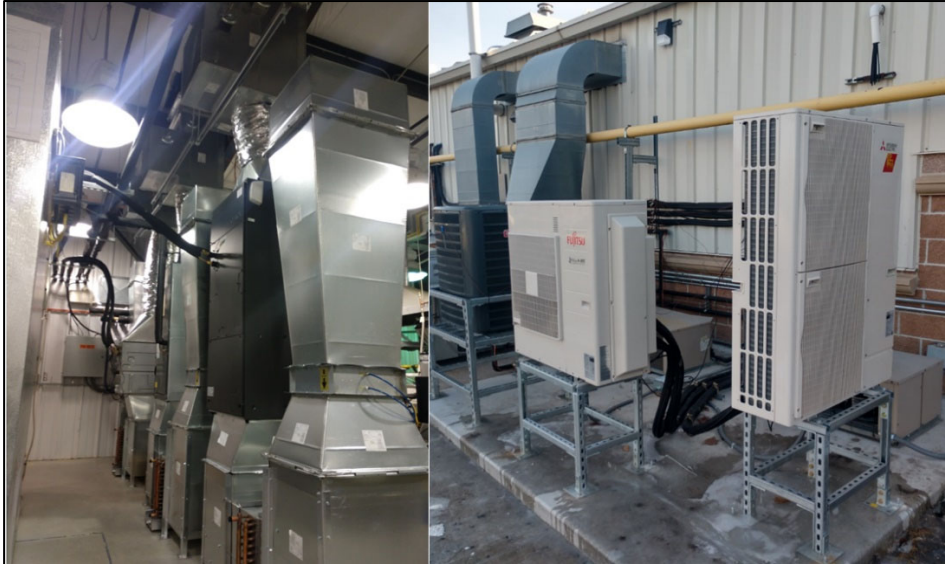
Figure 13 – Indoor (left) and Outdoor (right) ASHP Component Installations
